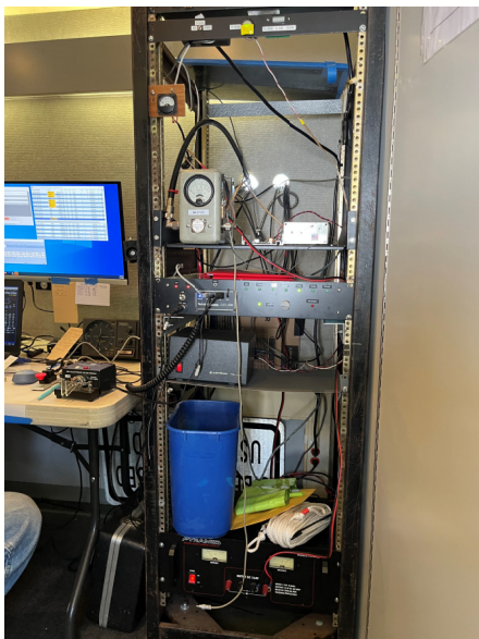
A portion of the \mu Wave equipment, other equipment was mounted at the antennas
