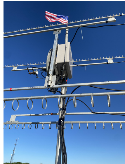
The completed microwave antenna array
